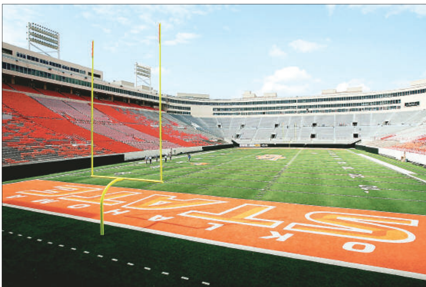
The west end zone of Boone Pickens Stadium is still under construction, but the stadium now holds 60,000. Completion of the west-end football complex is expected in August 2009. JAMES GIBBARD/Tulsa World
