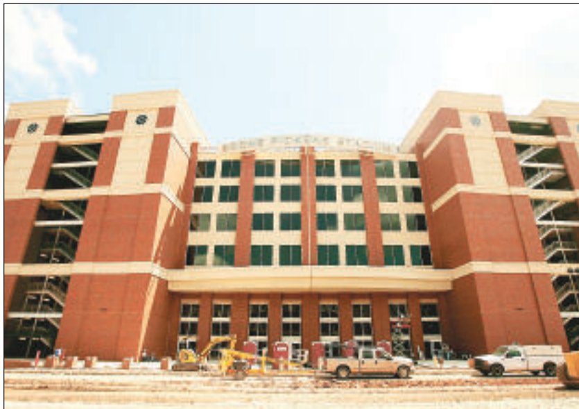
At 460,000 square feet, the west end-zone complex is larger than Oklahoma’s state Capitol. It is currently under construction. JAMES GIBBARD/Tulsa World
